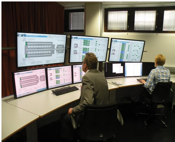
FIGURE 2.9: Example SCADA Control Room
